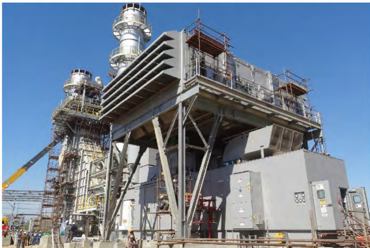
Co-generation Power Plant
